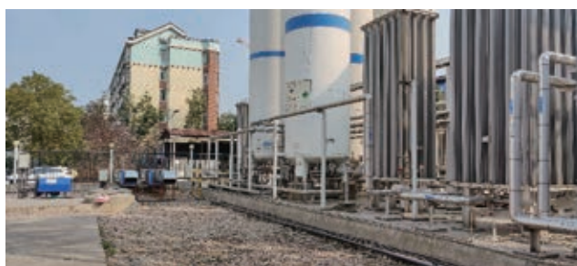
Carburetor spray water collection device
